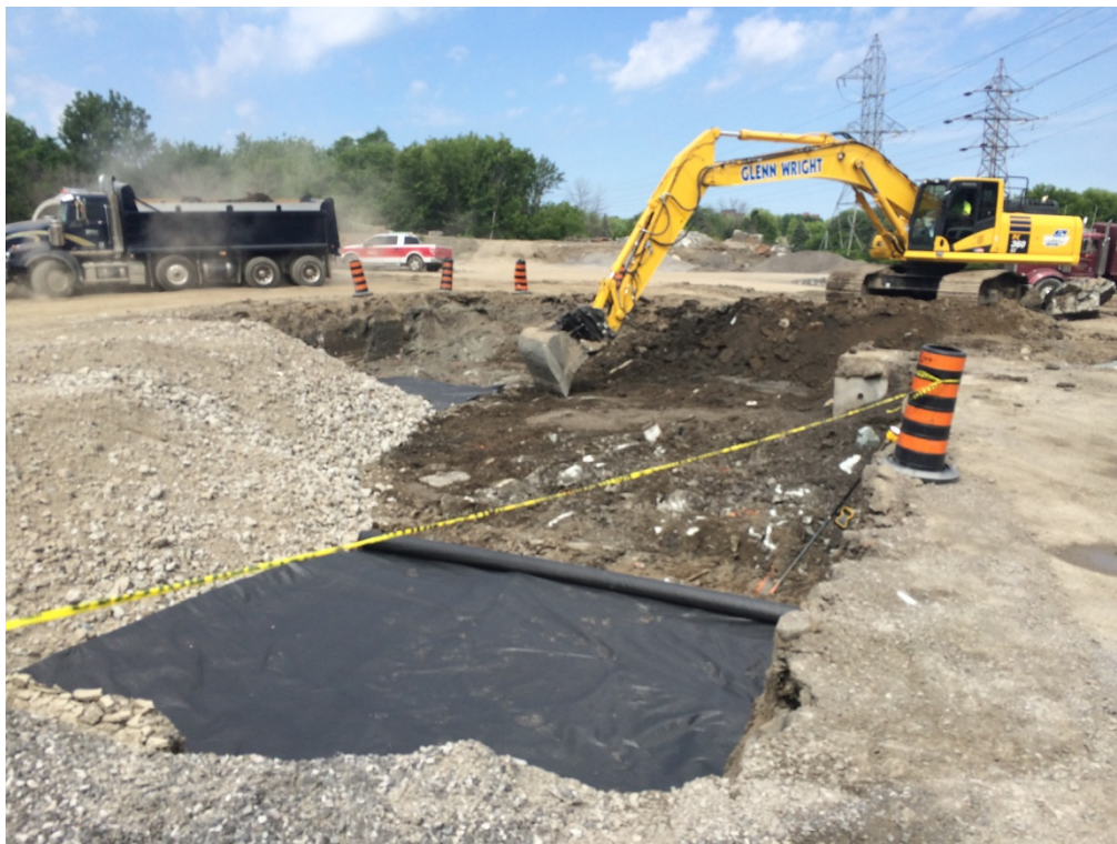
Excavation and placement of geotextile and select subgrade material for Frobisher Lane extension.
