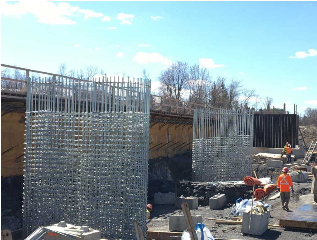
Construction of the VIA Bridge substructure footings and pier columns (shown facing south).
